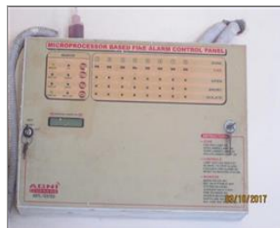
Photo of fire safety equipment Fire panel.jpg
