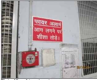
Photo of fire safety equipment Fire alarm.jpg
