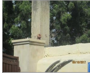
Photo of fire safety equipment Fire hooter.jpg
