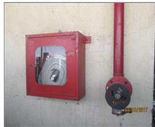
Photo of fire safety equipment Fire hydrant.jpg
