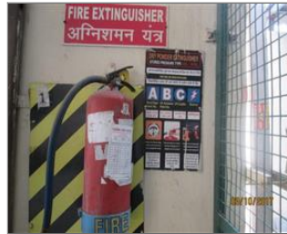
Photo of fire safety equipment Fire extinguisher.jpg
